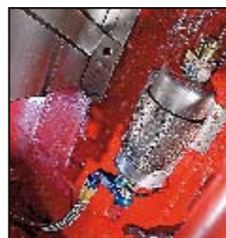
Be aware that old wiring will degrade over time
